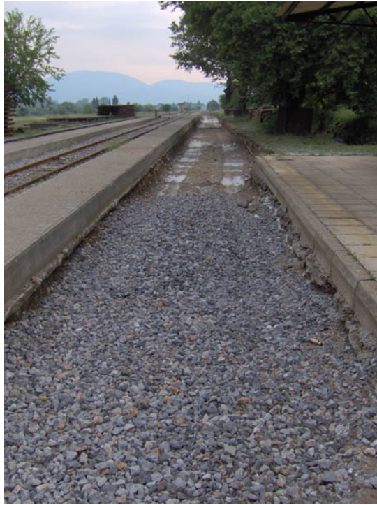
Here we have track 1 of Assea station. We can see that the track has been removed and the substructure is being renewed. (Photograph: Andreas Kapaklis, June 2005)
